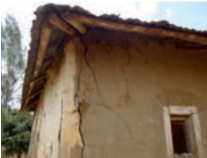
The mud house was in terrible condition.
